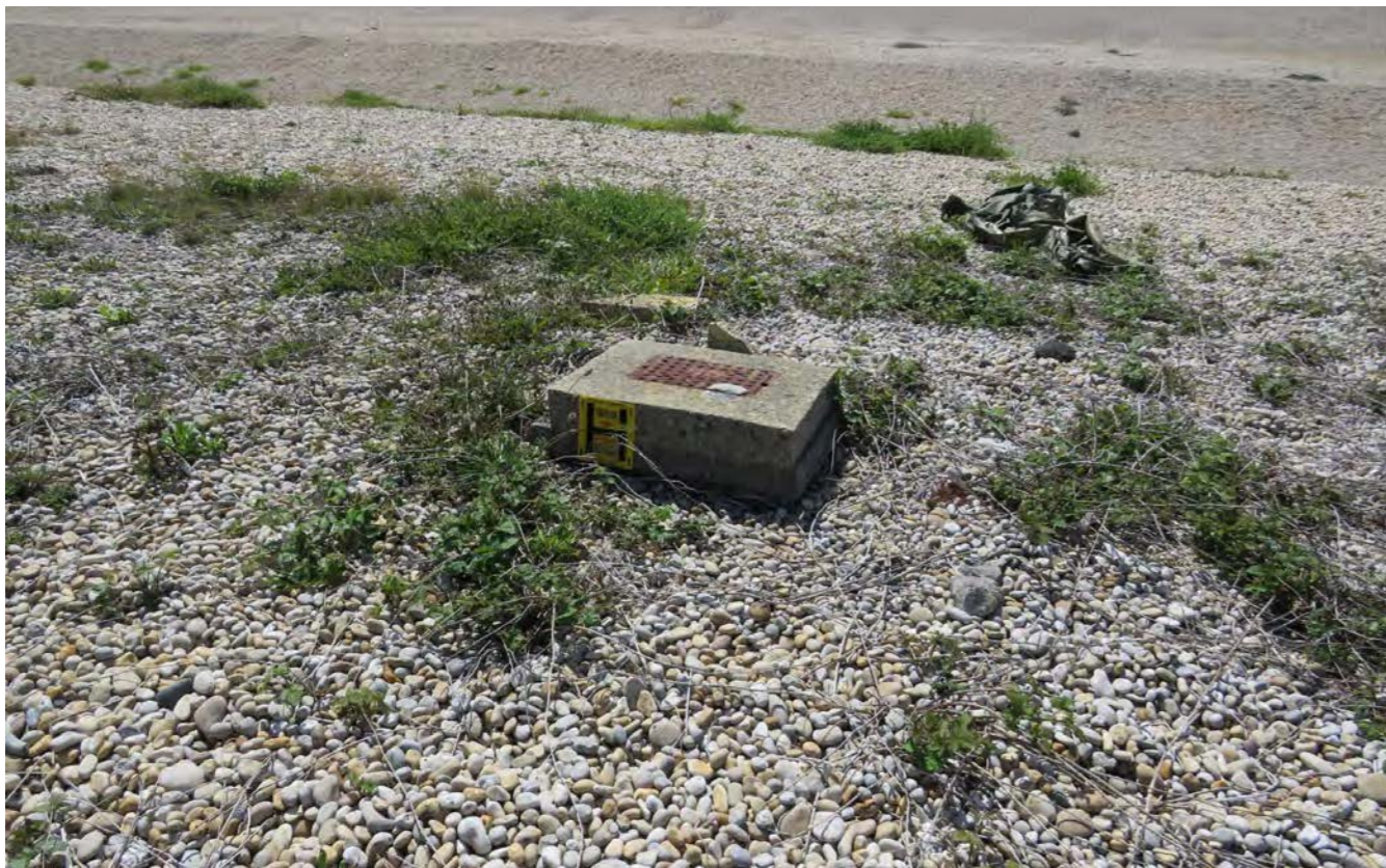
Photo 15: Evidence of utilities within vegetated coastal shingle habitat within Chesil and the Fleet SAC.
